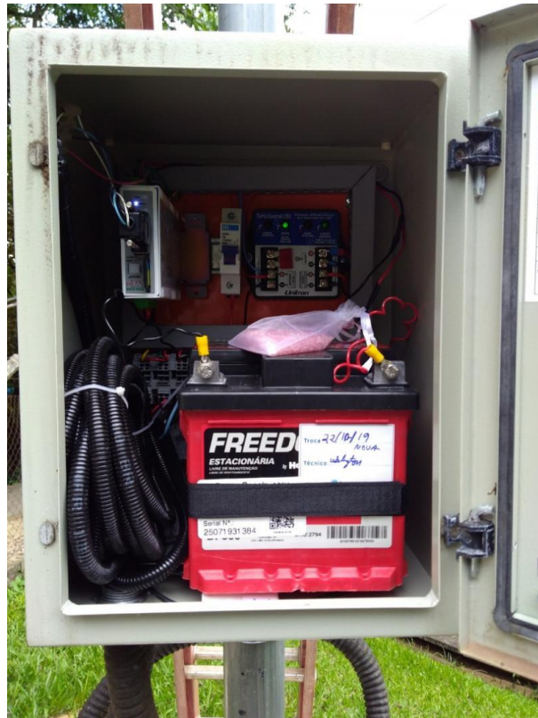
Interior do Painel
