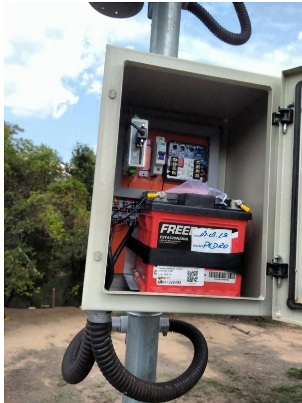
Interior do Painel
